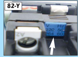
82-Y Tagged Coil Voltage Siemens
